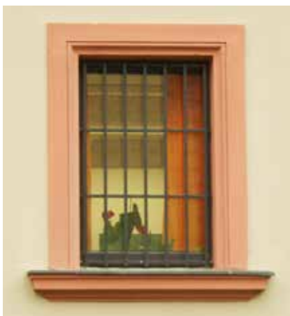
1 Fenstervergitterung (Copyright Thomas Steger).
